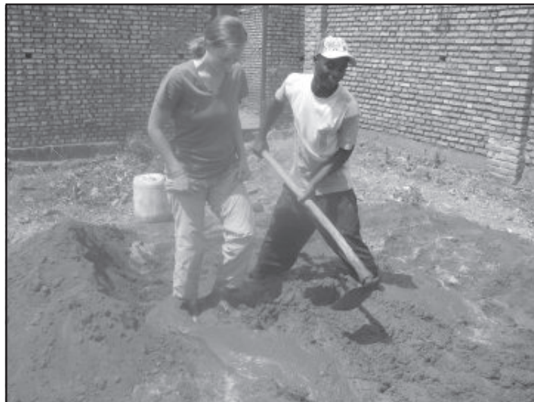
Work campers, Anna Considine and Martin Nahishakiye, play in the mud to make mortar for the clinic walls. Photo by Lin Considine
