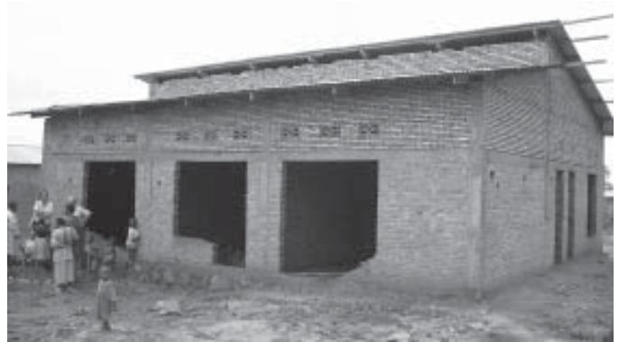
Friends Women's Association Kamenge Clinic built by AGLI workcampers in July 2006 as it looked in November 2006. Since this picture the FWA is finishing the center room—door, window, plastering walls, floor, and electricity—so that they can move in by April when the lease of their current building expires.
