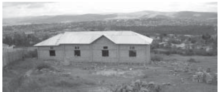
This was built by the July 2007 AGLI workcampers for the street children's program in Rwanda. The blocks were made by the older children who would like to make cement block-making into a business. Because of the considerable amount of firewood used to make bricks, the government has banned the use of bricks.
